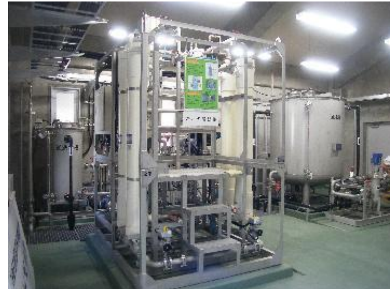
Membrane filtration facilities, Water supply system for Kuroda area in Kyoto city, Waterworks Bureau, City of Kyoto
