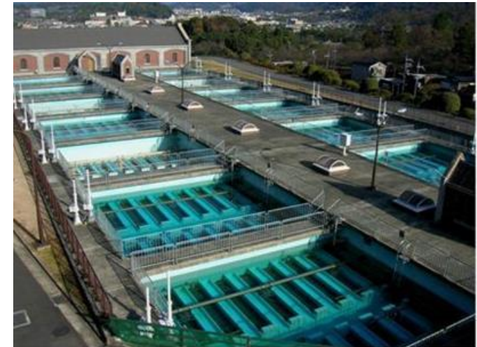
The first plant using rapid sand filtration in Japan (Keage WTP, Kyoto City)
